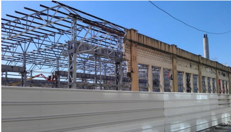
Photograph 2. The Alstom hall being turned into the city of design (Saint-Ouen). Source: G. Djament, May 2015.
